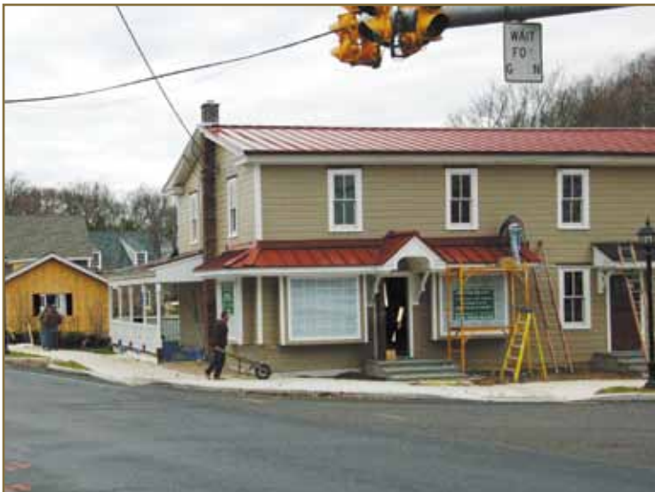
Work is under way to revitalize historic Edgewood Village into a town center for Lower Makefield Township.
