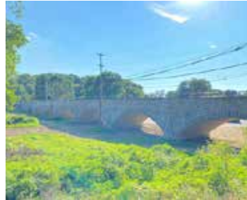
Restoration of the Rt. 52 (Lenape Road) Bridge crossing the Brandywine Creek Floodplain.
